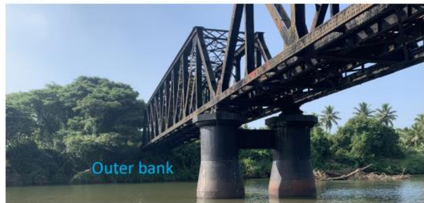
Aggressive meandering at a critical location (Railway bridge, Manuwangama) along Deduru oya
