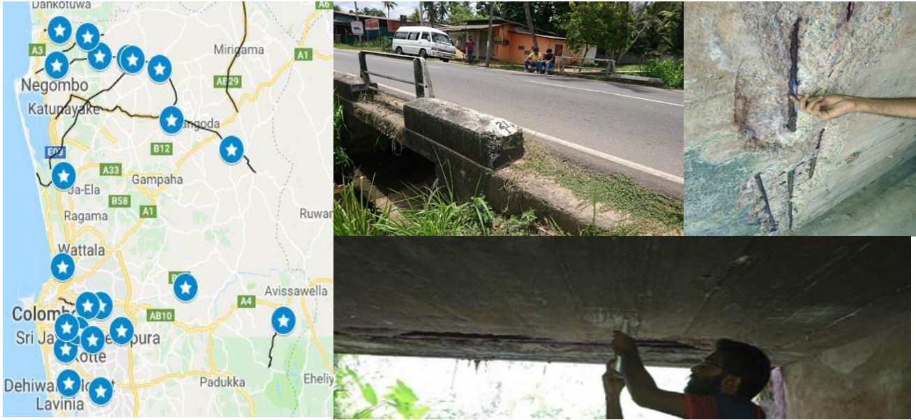
Locations of the conducted bridge inspections and observations during a bridge inspection
